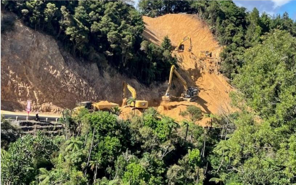
Figure 7. Another slip on Sate Highway One over the Brynderwyns, 2024. Toe sloep cuts destabilise the already unstable regolith. Image: NZTA.
